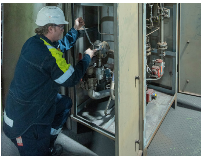
Primetals technician at SIP box (source thyssenkrupp AT.PRO tec GmbH)
