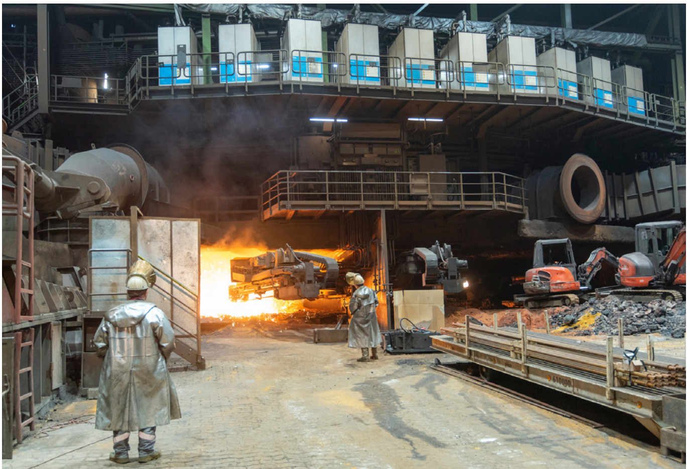
A blast furnace with SIP installed. The proprietary SIP boxes can be seen in the upper part of the picture (silver/blue) (source thyssenkrupp AT.PRO tec) GmbH
